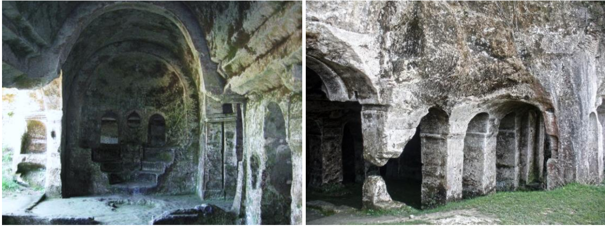
F. 19: Bema, apse, synthronon and cathedra F. 20: Deterioration of the north side cell and side nave (Mısırlı, 2019)
